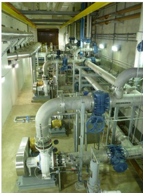
Figure 3-2 Pump Gallery of an ATAD Installation in Colorado
